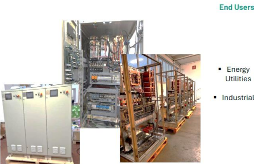
Figure 27: SCR Converters (Battery charge)
